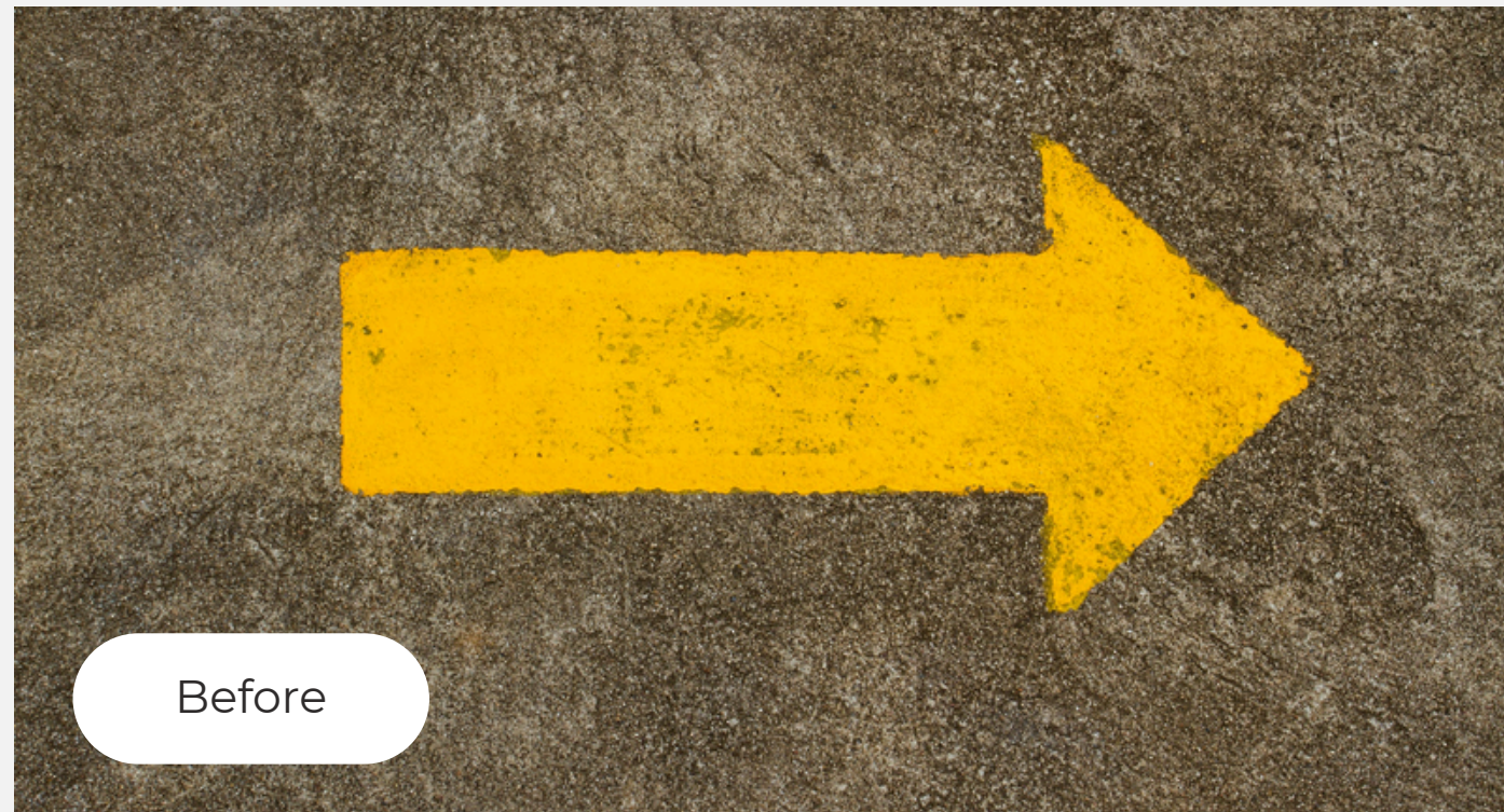
Outdated safety signs
